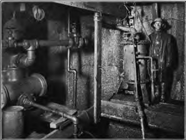
PLATE 1. SHOWING GROUT MACHINE AND CONNECTIONS. FOUR INCH SUPPLY PIPE FROM SURFACE EMPTYING INTO TANK.
